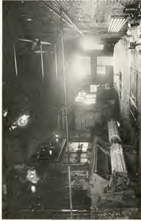
The Boiler Room—Bloomington Water Works
